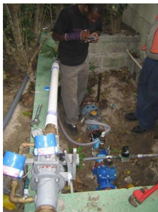
Checking accuracy of a large customer meter.
