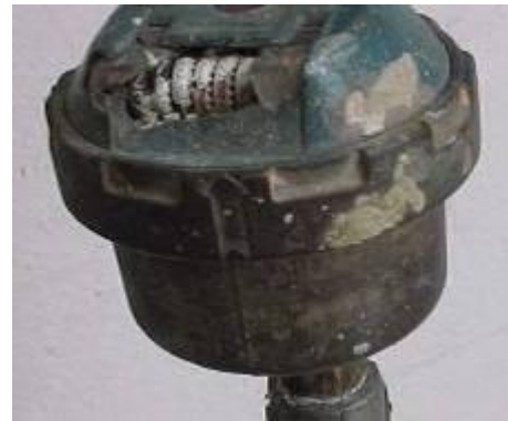
The customer has tampered with the meter's moving parts.
