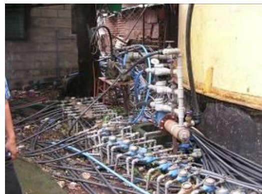
Improper meter installation leads to inaccurate data and billing errors. Meter readers in the pictured situation will find it difficult to determine which meter belongs to which property.
