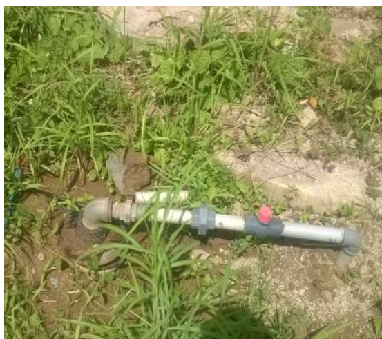
Figure 3.53. Inadequate protection of pumping mechanism at Rehab. Centre, Bwari, FCT
