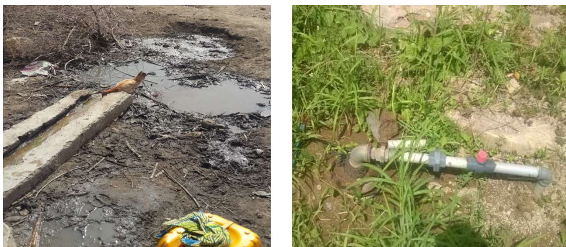
Figure 3.64: Very poor sanitary status at pumping surrounding and inadequate protection of supply pipe
