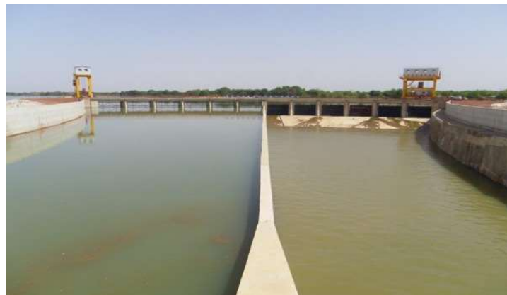
Regulating Felou dam
