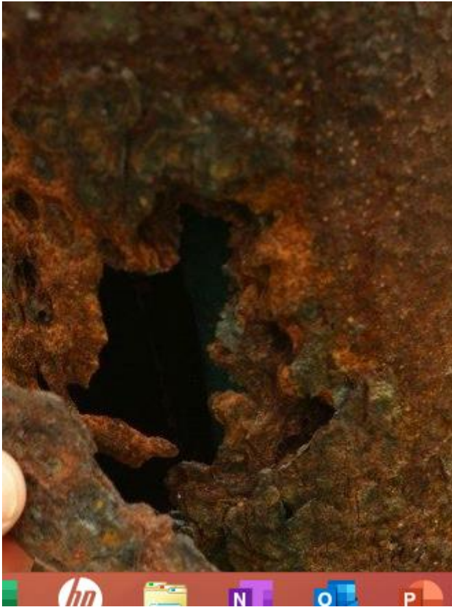
(Fig. 5.2). Tube well due to corrosion The other indication is increase in sand pumping,
