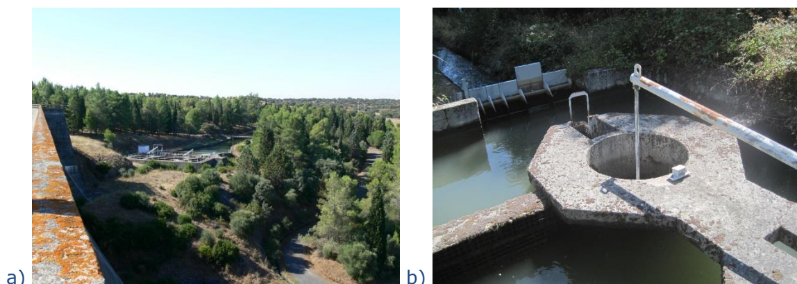
Figure 2. Example of pressure reducers installed at the dam toe, upstream irrigation networks: a) Odivelas dam; and, b) Gostei dam, both in Portugal.
